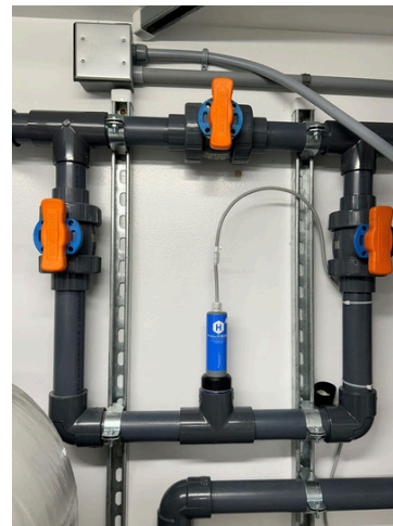
Figure 13. Upward-flowing field installation.
